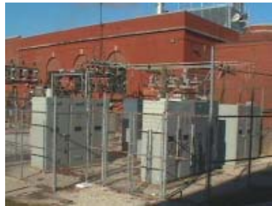
Power Plant Substation
