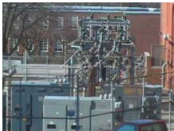
ISU High Voltage Electrical Station
