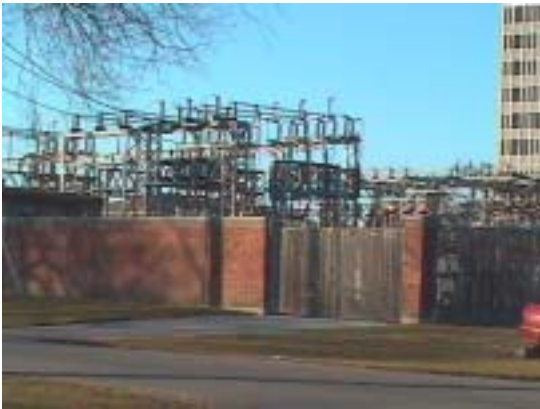
Osage Street Substation
