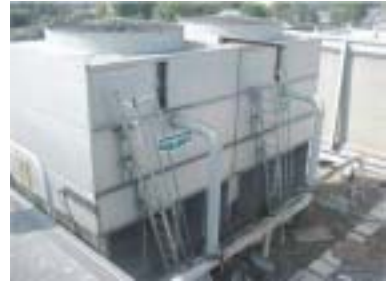
CVA Cooling Tower
