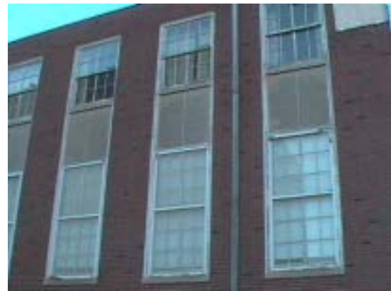
Loss of Energy due to need for Window Upgrades
