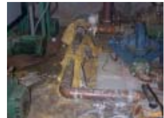
Poor Insulation in Mechanical Rooms
