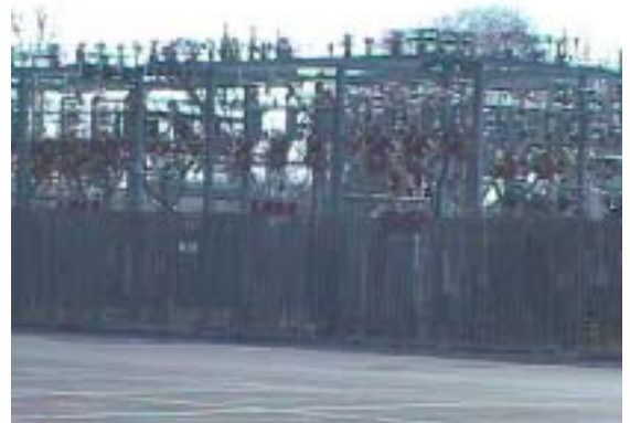
Osage Street Substation
