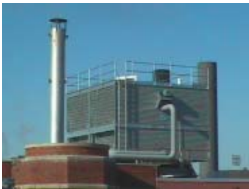
ISU Power Plant Cooling Tower
