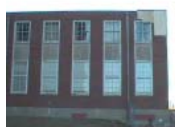
Inefficient Bldg Envelope
