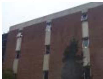
Windows Open in Heated Facility
