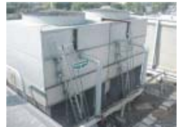
A non-metered Cooling Tower
