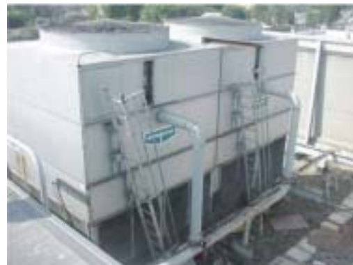
CVA Cooling Tower
