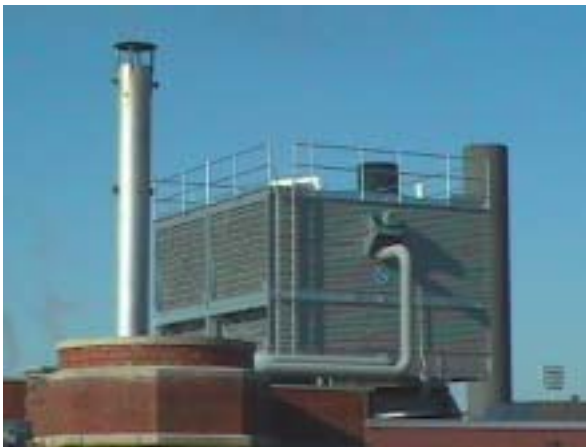
ISU Heating Plant Cooling Tower
